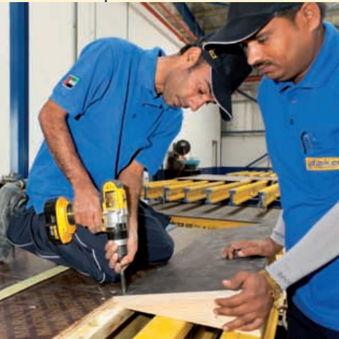
▲ Ready-to-Use is by far the most effective method of speeding up a formwork project.
