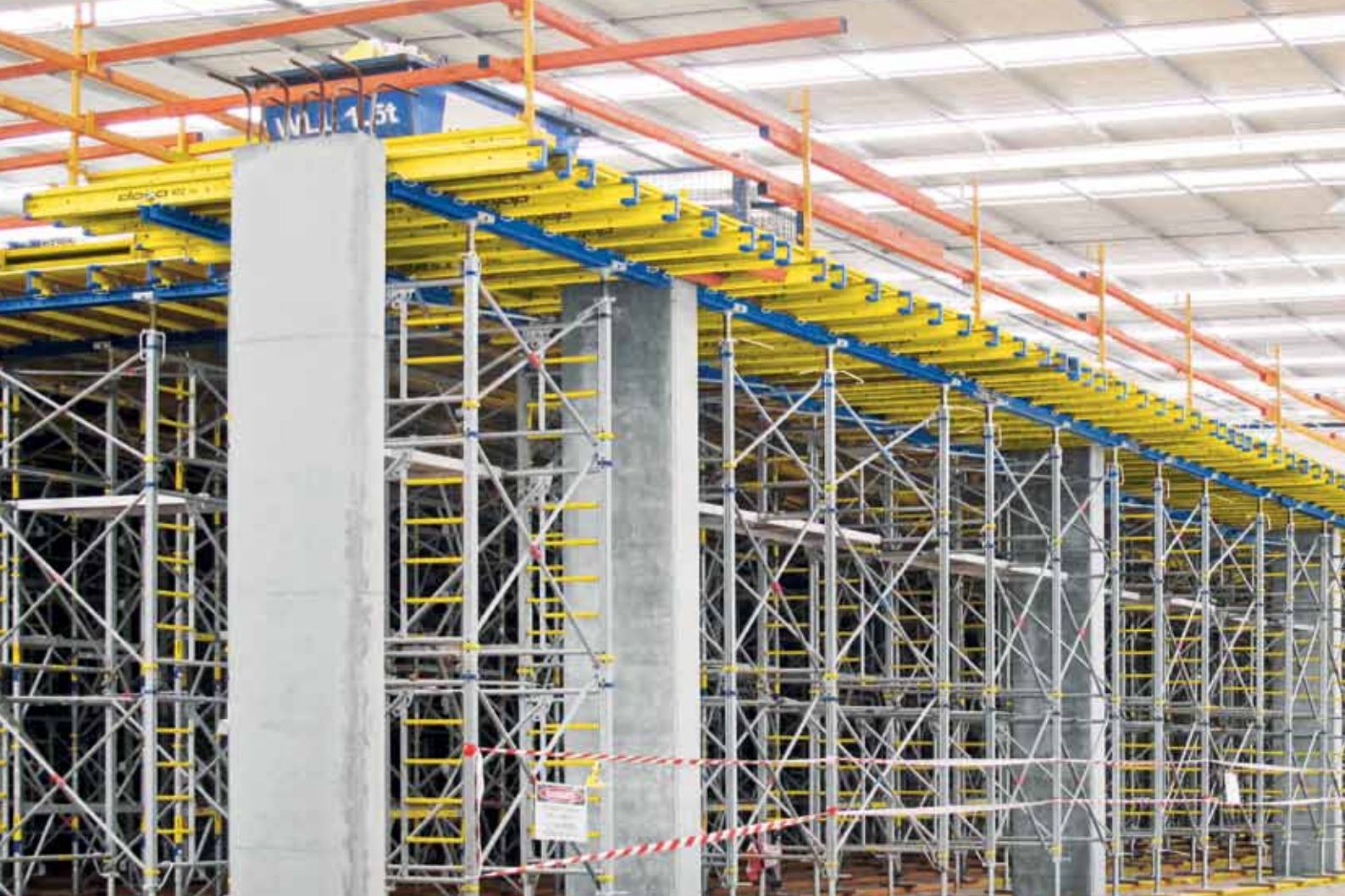
▲ Large quantities of load-bearing towers Staxo 100 and Staxo 40 were erected quickly and safely.
