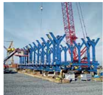
▲ Preparations for the immersed Second Midtown Tunnel are underway in the dry dock.
