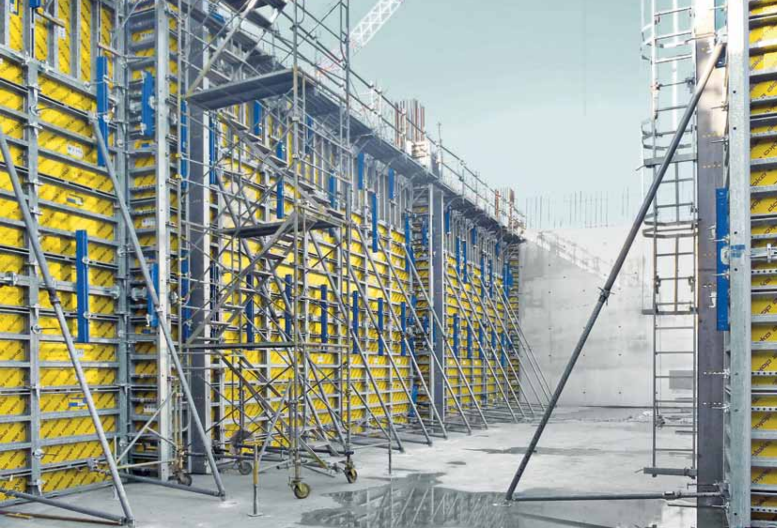
▲ The total area of formwork used was 1,700 m 2 – for six rotations on each floor in a 4-day cycle.
