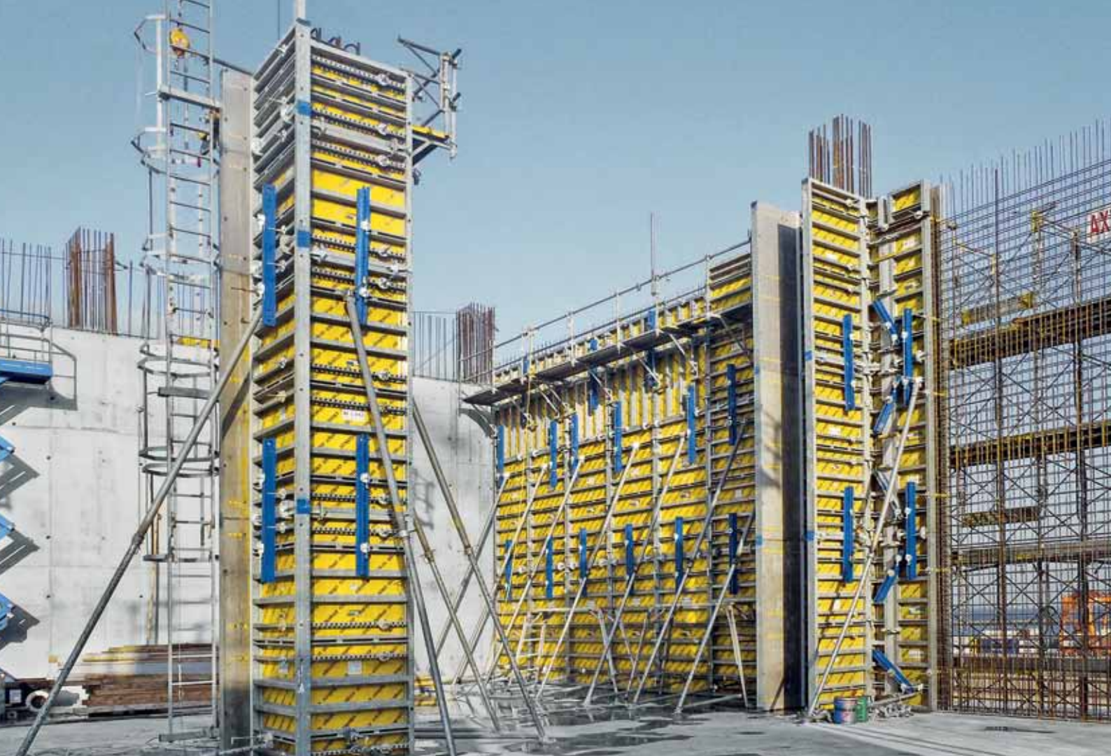
▲ Doka Japan was chosen to supply column and wall formwork for a project to build a large refrigerated warehouse in reinforced concrete.
