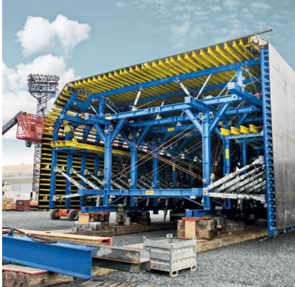
▲ The combination of the high-performing 'heavy-duty supporting system SL-1' tunnel formwork and Large-area formwork Top 50 is ideal for the box cross-section of the eleven tunnel segments for the immersed Second Midtown Tunnel.
