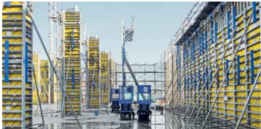
▲ Doka gained a high reputation by implementing eight Framax column formworks and 1,400 m 2 of wall formworks.
