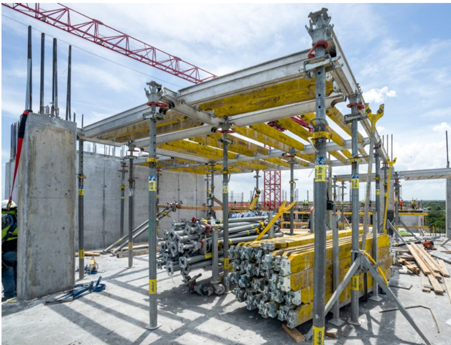
Bay by Bay: The 8' × 8' grid pattern spans across multiple bays, showcasing SuperDek's efficiency in forming large floor areas with minimal props and simplified logistics.
