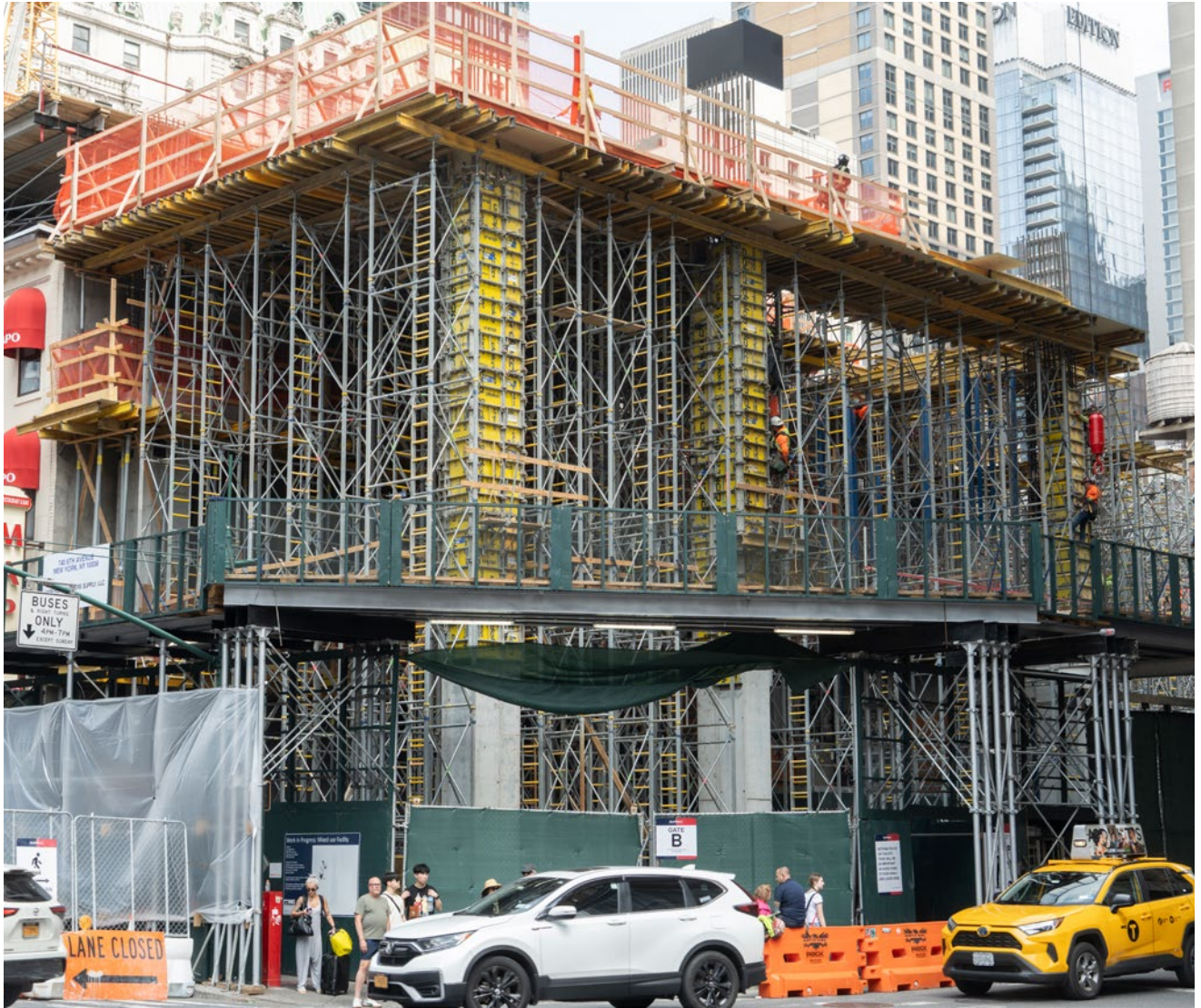
Coordinated Systems: Interior platforms, wall formwork, and shoring work in concert as The Torch transforms Manhattan's skyline.
