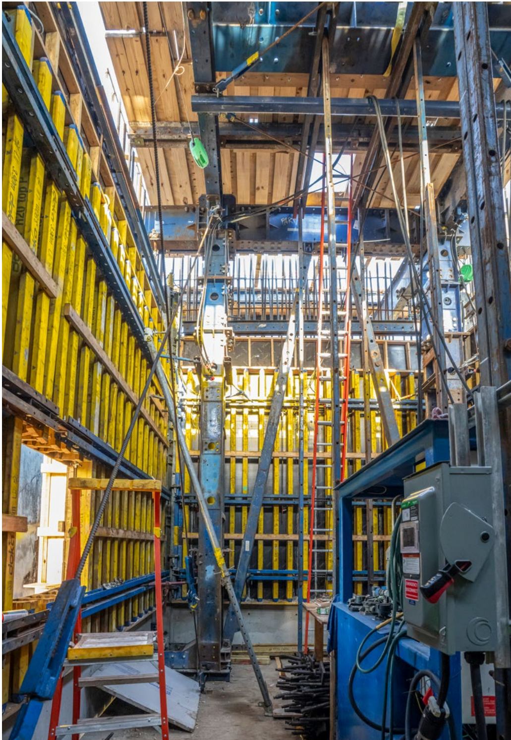
Inside Efficiency: Interior view of the Super Climber SCP platform above the working deck, providing safe access for crews during core construction.
