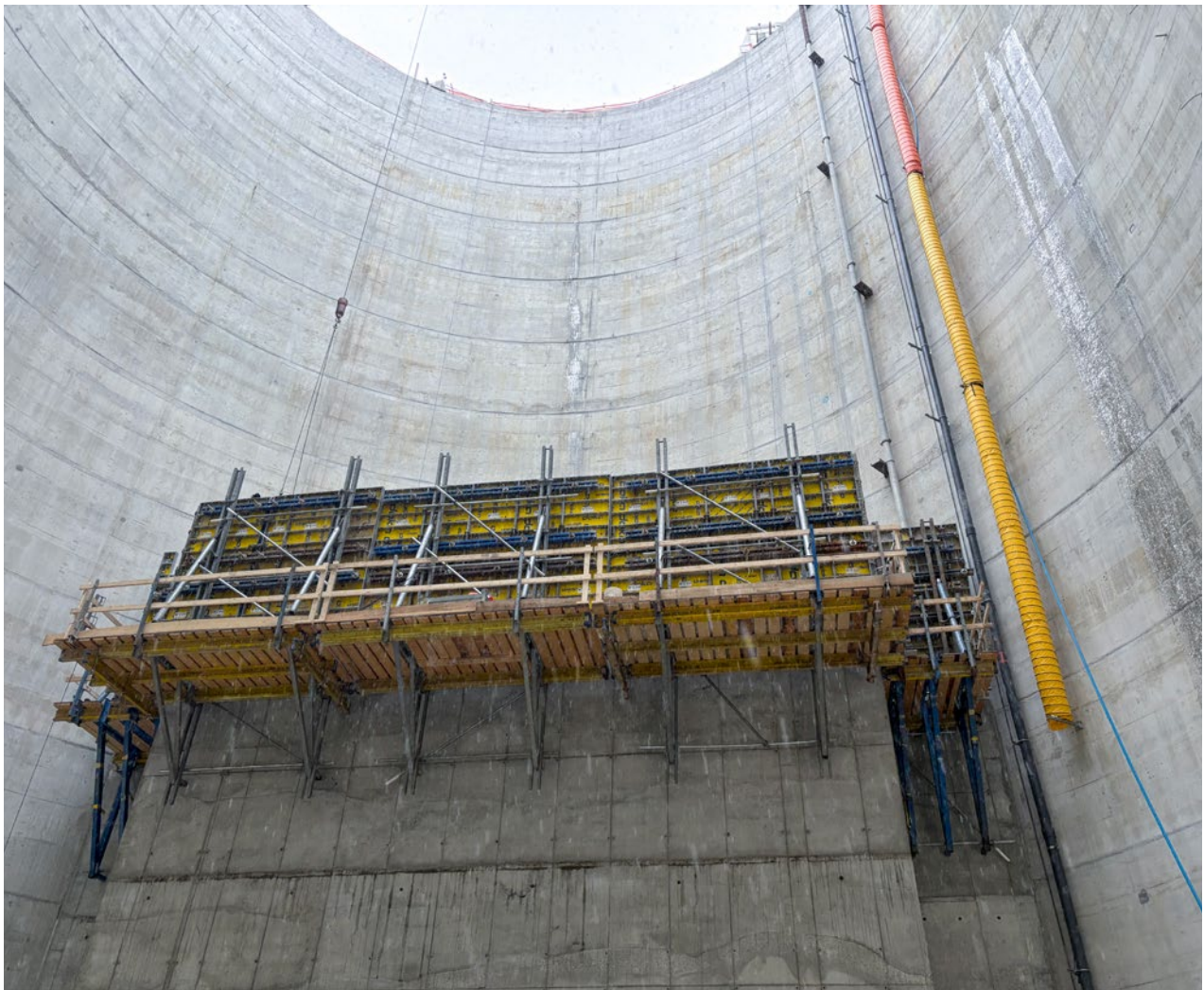
Safety and Structure Combined: Inside the circular shaft, Doka MF240 climbing formwork works in tandem with D22 construction supporting frames to enable efficient vertical progression.
