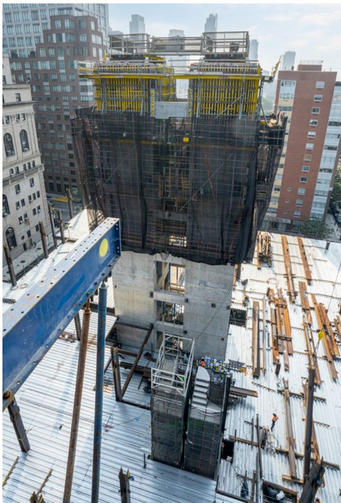
Platform Power: Doka's Xclimb 60 system supports formwork from below, enabling independent climbing operations on the East Core while maintaining cycle efficiency.
