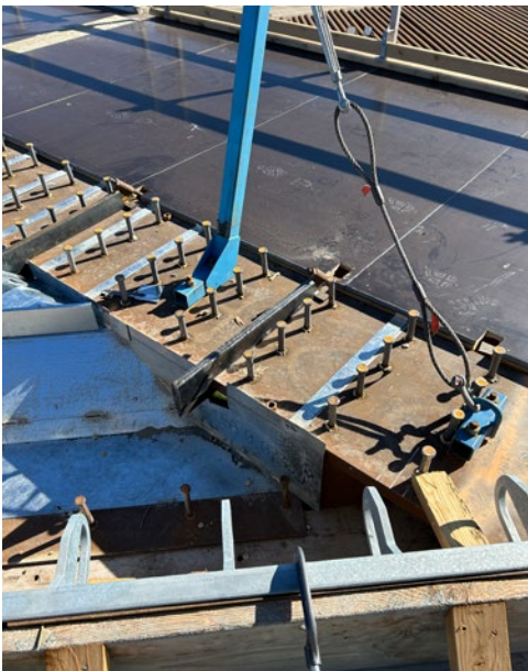
Custom Fit: Close-up of the redesigned C-130 Dayton hangers showing the laser-cut modifications that resolved rebar conflicts while maintaining full structural capacity.
