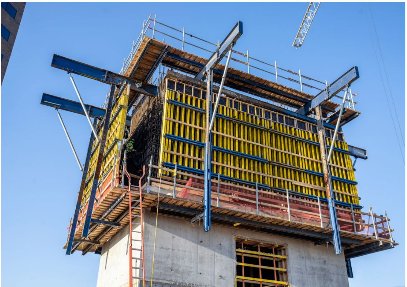
Automatic climbing formwork solution: The Super Climber SCP on the main elevator core climbs independently without crane assistance, freeing the tower crane for other critical lifts.
