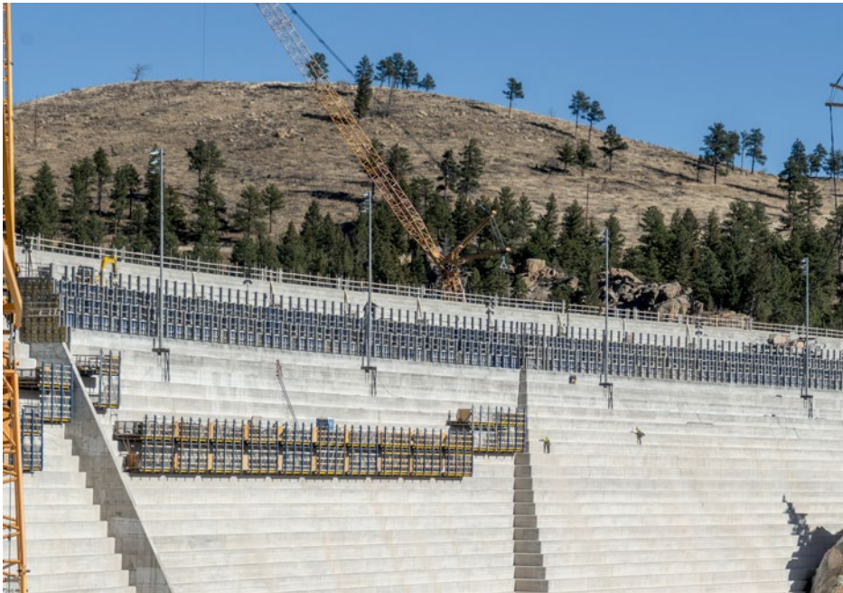
Form Fit: The crew used Frami formwork on the upper training wall (visible at top left) to better facilitate pours during challenging winter conditions.
