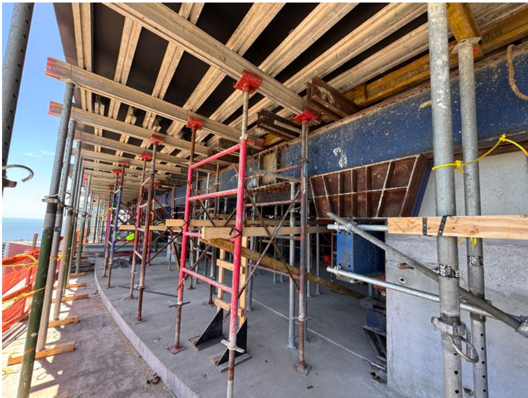
Easy Load Distribution: A belt wall with 140-kip jacks distributes heavy wall loads while maintaining reshore-free construction below Level 37.
