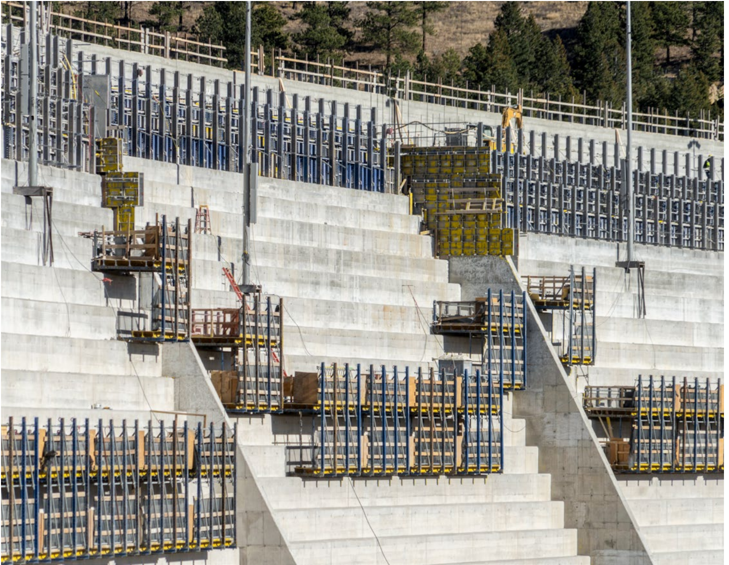
Lift and Load: Forms are assembled to allow three 4-foot lifts before repositioning for the next sequence.
