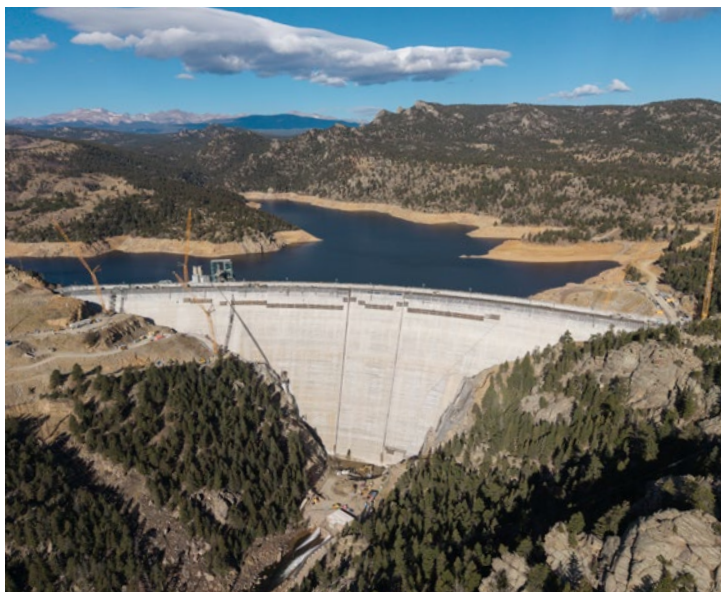
Heavy Pour: Throughout construction, crews have been placing over 3,000 cu. yds. per day.
