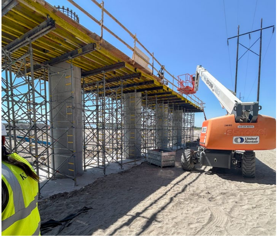
Strength in Numbers: The bridge formwork must support multiple load conditions throughout construction.
