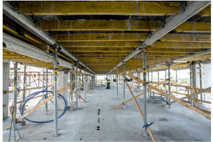
Adaptable Assembly: Crews rapidly formed typical bays using joists and stringers that adjusted around cores, offsets, and mechanical zones—no specialty parts required.
