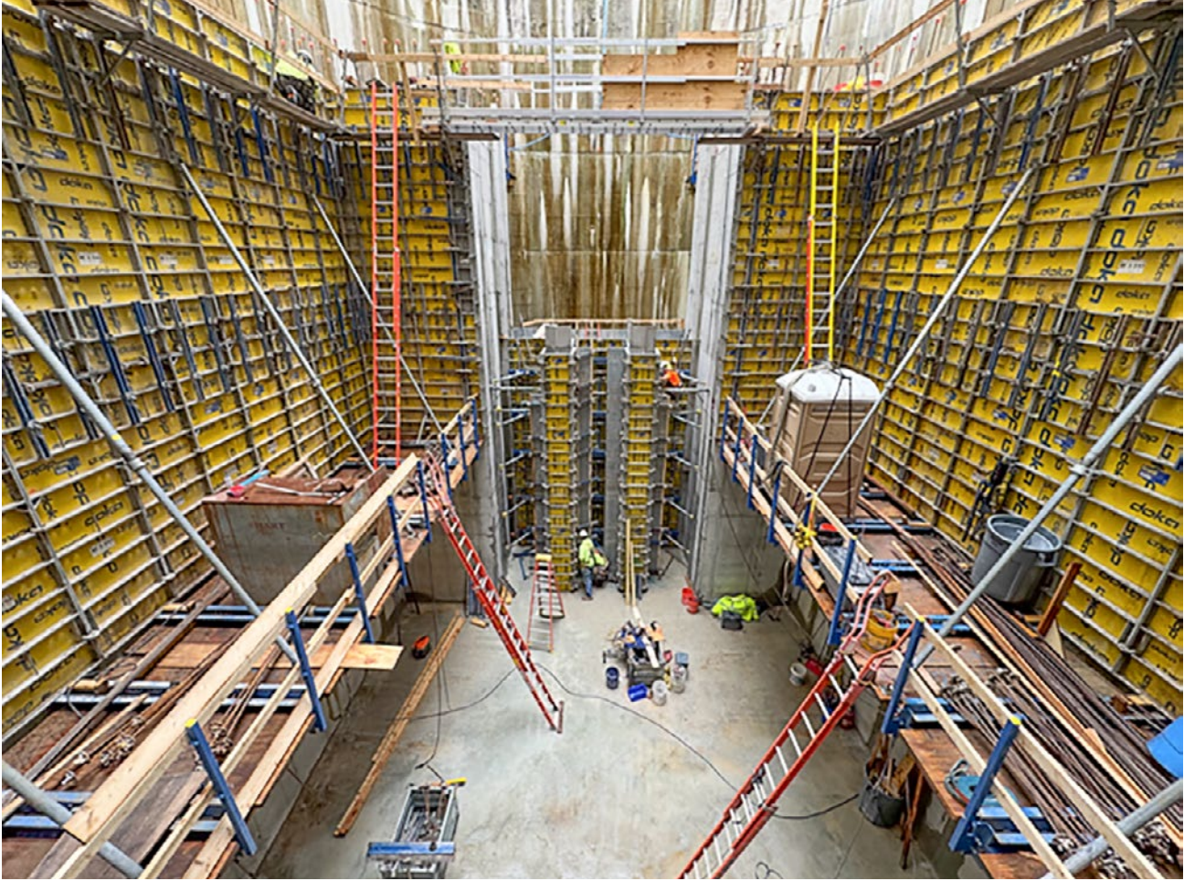
Versatile Wall Forming: The Doka Frami Xlife modular system adapted easily between the different shaft configurations—critical for a project with varying dimensions from 273 sq. ft. to 3,100 sq. ft. per pour.
