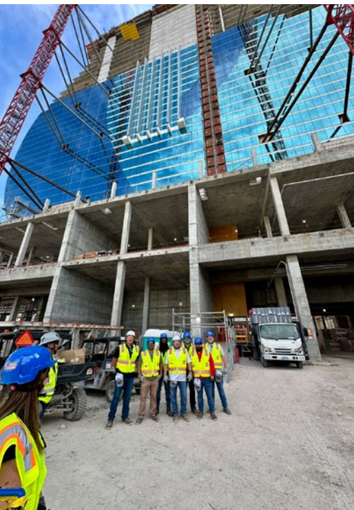
Customers had the opportunity to visit a nearby landmark project and see Doka climbing systems in real-world operation.
