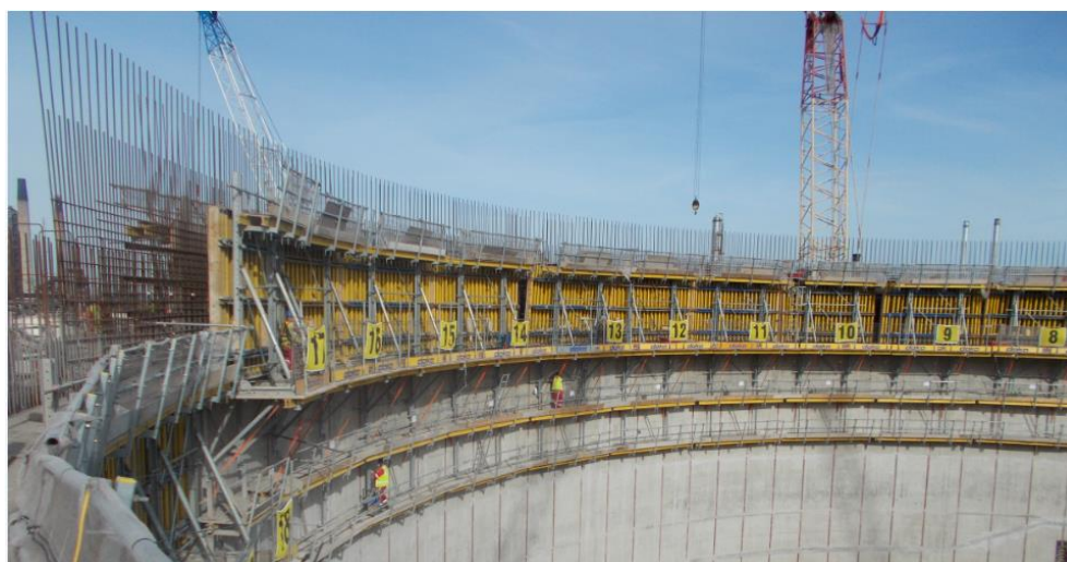
Doka Top 50 circular formwork, including MF240 Climbing brackets + 2 minus level working platforms
