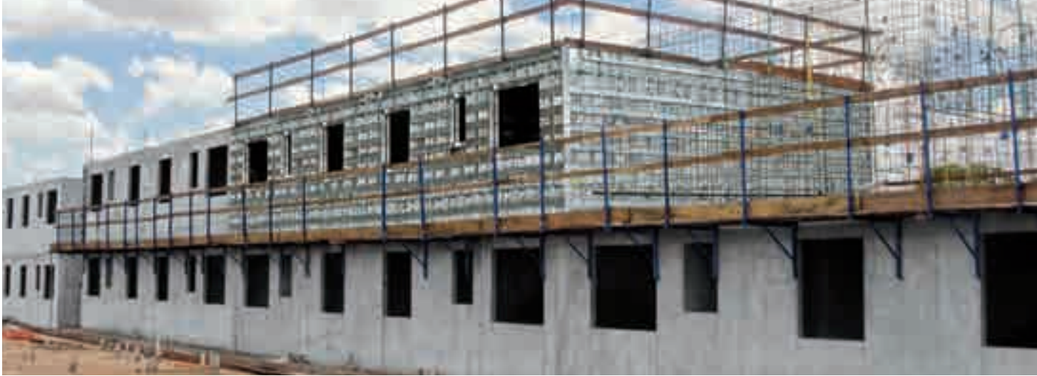
▲ Construction works are well underway and have already reached the second level.
