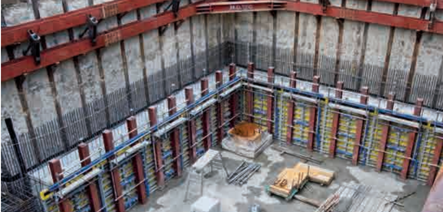
▲ Using earth retaining members instead of supporting construction frames Doka established a new construction method.
