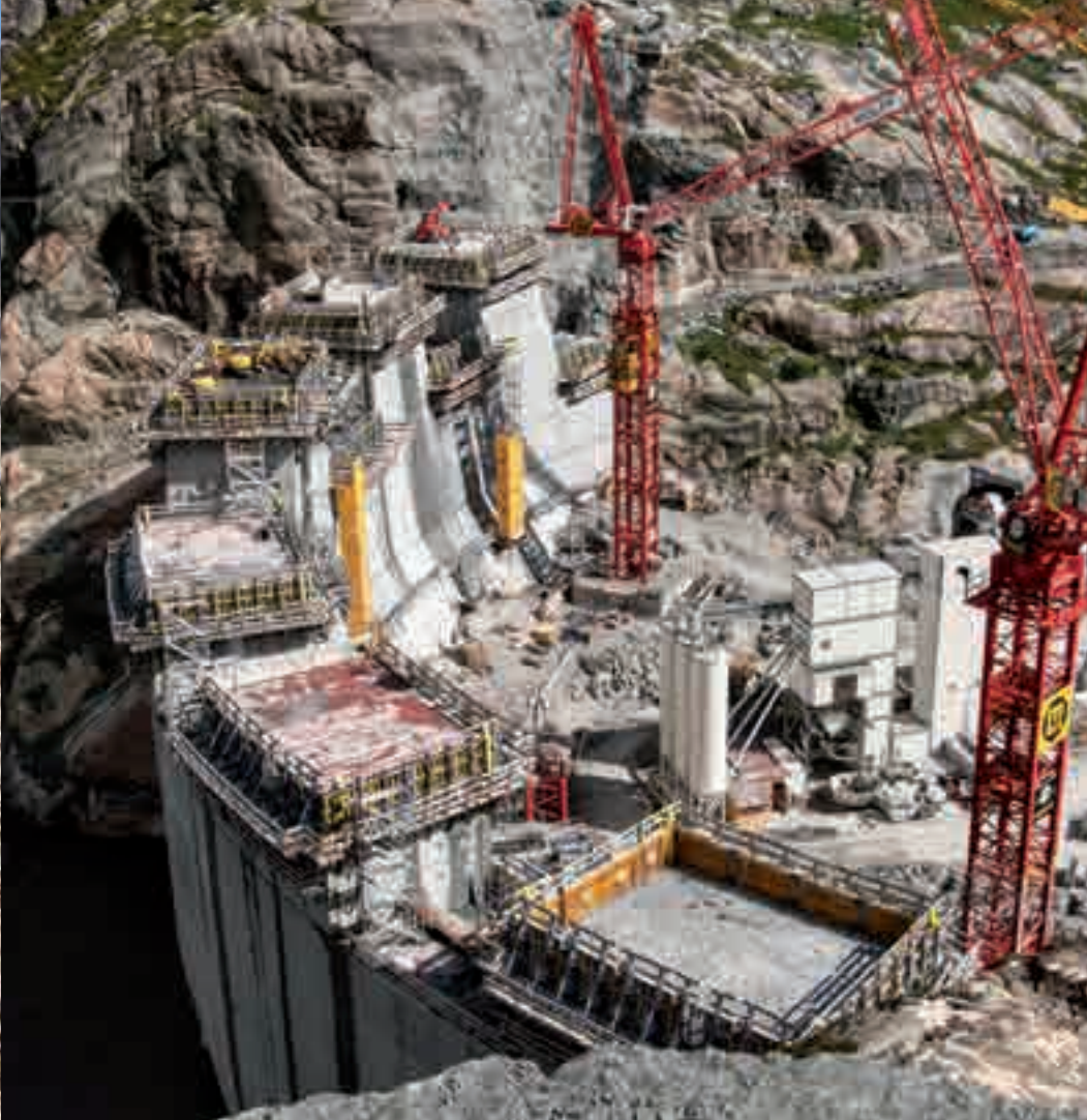
▲ The gravity dam exhibiting a roughly 170 m long crest is built with the tried and proven Dam formwork D15 from Doka.
