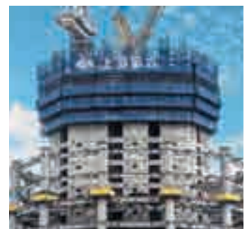
▲ Fully enclosed protection is installed above 0-floor platform and ensures safe working-conditions.
