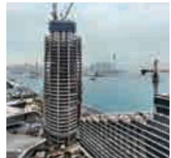
▲ Combining Automatic climbing formwork SKE50 and SKE100, Doka fully satisfies the client's various requirements for construction.
