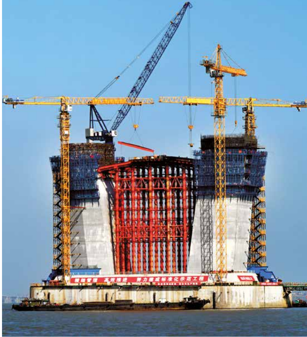
▲ Doka formwork solution for 6 m regular step height shortening the construction progress.
