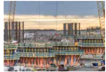
▲ Because it is so versatile, Large-area formwork Top 50S is the ideal solution for the straight walls and tight radii characteristic of the spillways.
