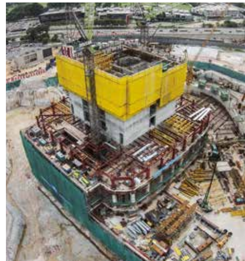
▲ The building core is divided into two sections and is being built with Automatic climbing formwork SKE100 plus and SKE50 plus. The entire outside of a section can be repositioned in a single operation with hydraulic cylinders.
