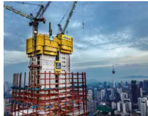
▲ Forward-thinking formwork planning – right from the start the cranes were taken into account in the formwork concept. So now they integrate seamlessly. Doka also supplied all the illuminated logos.
