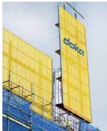
▲ All gaps are closed off to prevent tools or small things being dropped, thus providing a safe work environment.
