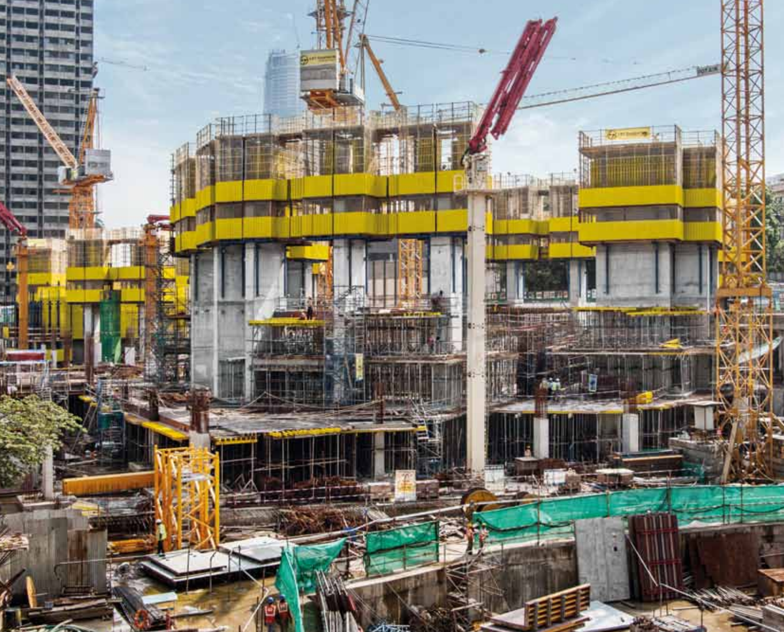
▲ Wall formwork Top 50 was designed to perfection in order to obtain the concrete pattern designs set by the architecture.
