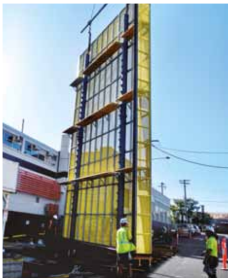
▲ Safe working conditions during construction of the Trafalgar Lane project are assured by the Protection screen Xclimb 60.
