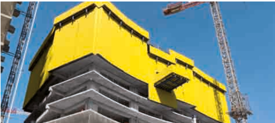
▲ Protection Screen Xclimb 60 enables safe and weather shielded working conditions while the self-climbing system SCP moves the formwork automatically.
