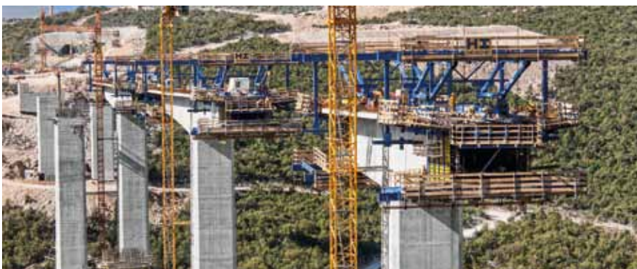
▲ For construction of the bridges spanning 555 m and 365 m in length, Doka developed a formwork solution consisting of Cantilever forming travellers that saved time and resources thanks to extended pouring sections.
