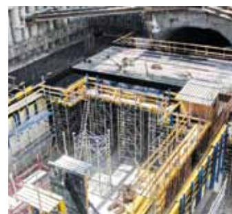
▲ Even architectural demands such as with the Metro expansion in Algeria are realised quickly and safely with high-performing Doka products.
