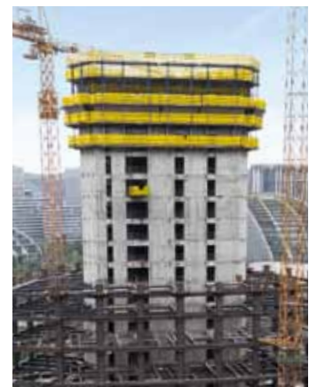
▲ Doka supplies Automatic climbing formwork SKE50 and Large-area formwork Top 50 for the project, cutting down on tower-crane time and speeding up progress on the build.
