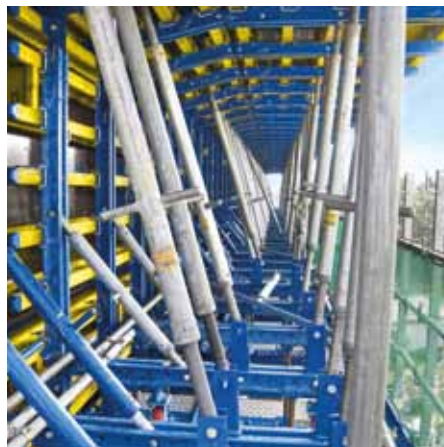
▲ Slab and sidewall formwork are made up of Large-area formwork Top 50, designed to take the weight of the concrete and be usable as a working platform to enhance safety.
