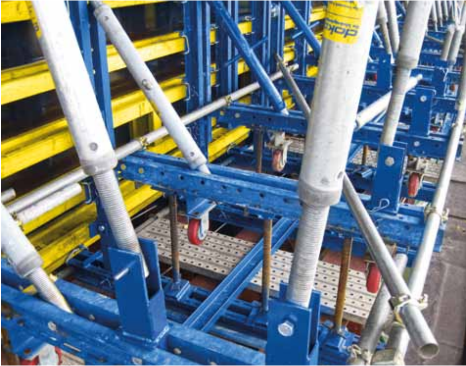
◀ The formwork for sidewalls and deck slab was designed to advance on rollers. There is no need for a crane, so site efficiency is enhanced.
