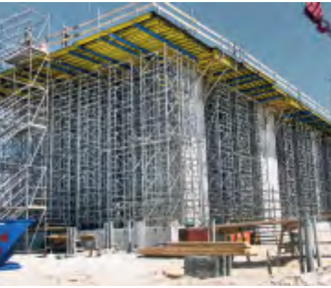
▲ Heavy duty shoring is offered on this substructure by Load-bearing Staxo 100, which is specifically designed for large shoring-heights and high loads.
