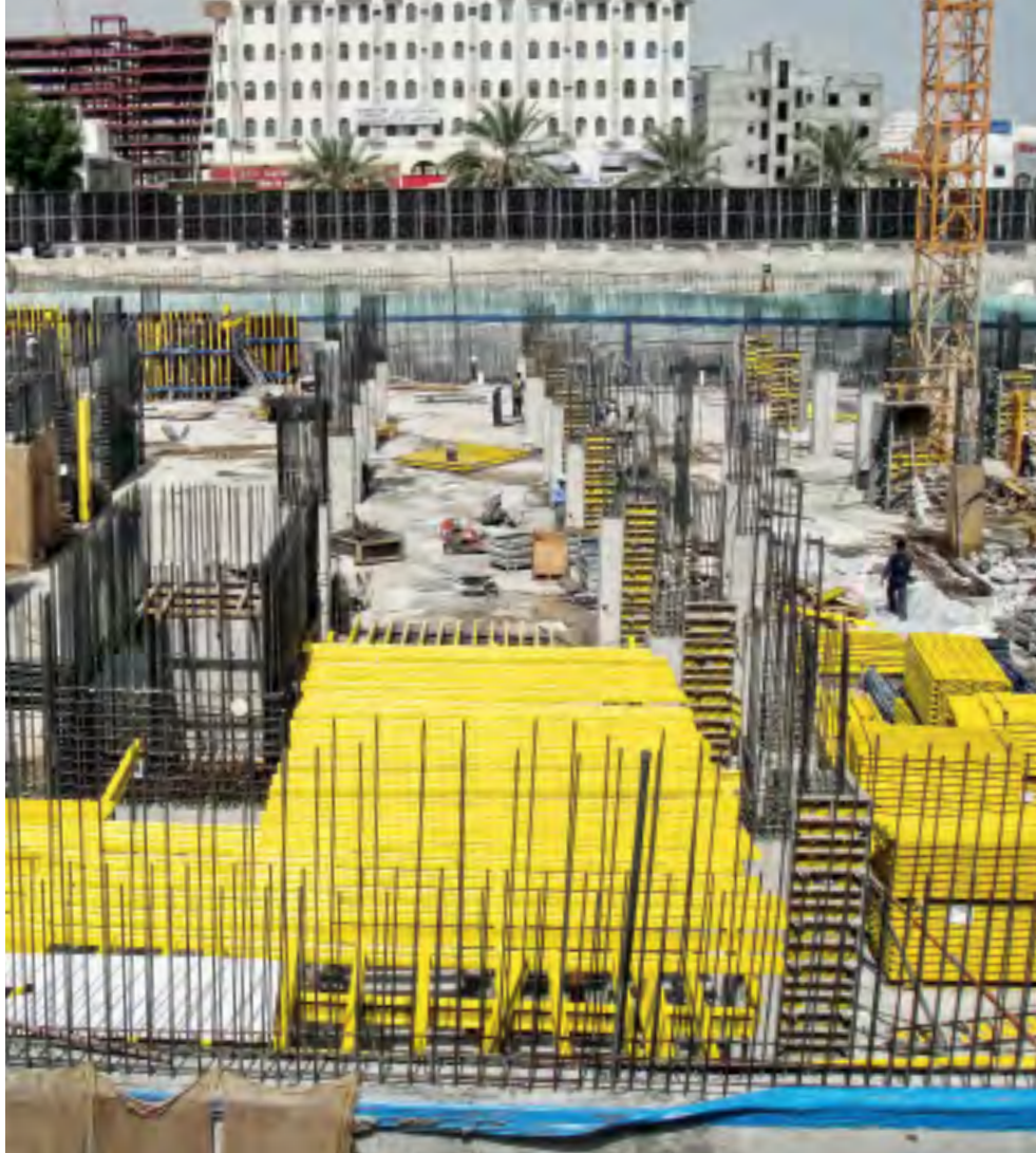
▲ From the initial stages Doka has contributed significantly to speed and safety onsite with supply of key systems.
