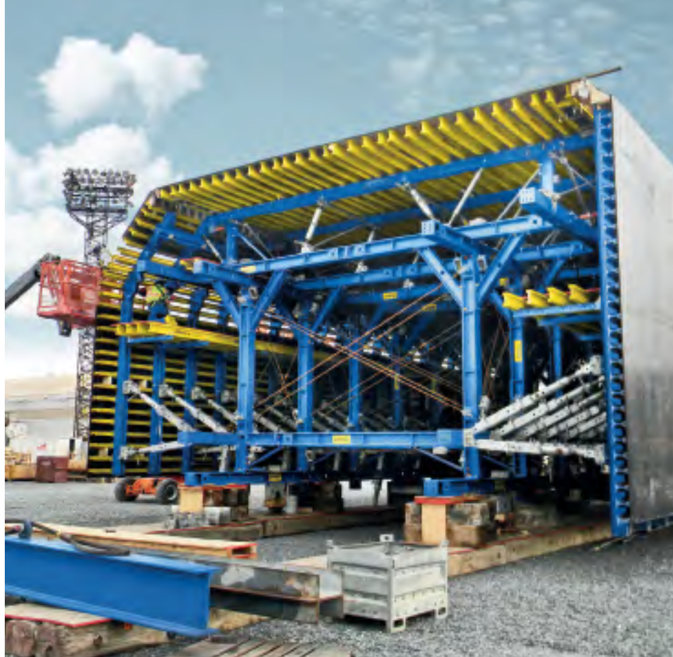
▲ The combination of the high-performing 'heavy-duty supporting system SL-1' tunnel formwork and Large-area formwork Top 50 is ideal for the box cross-section of the eleven tunnel segments for the immersed Second Midtown Tunnel.
