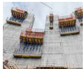
▲ Premiere for Dam formwork D35: the new Doka standard system is used for the first time during construction of the barrage "Dam Sarvsfossen" in Norway.
