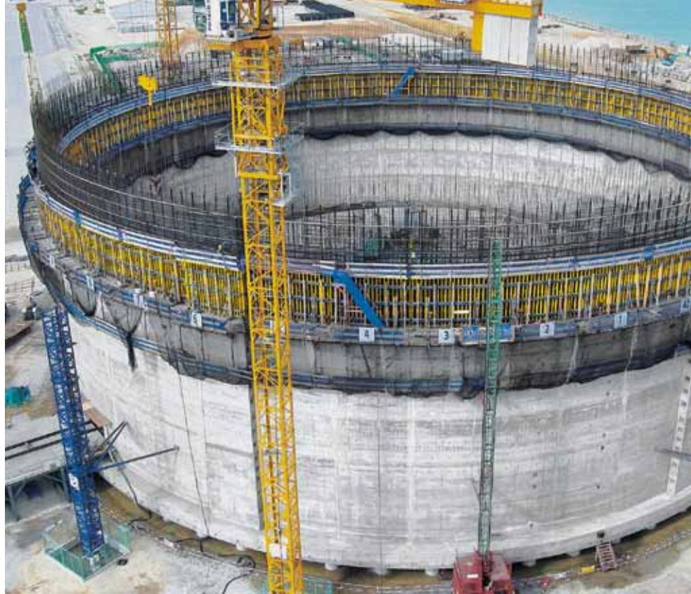
▲ The crane-lifted Climbing formwork MF240 ensured systematic forming processes as well as rapid construction process during construction of the LNG tank Map Ta Phut in Thailand that measures 82 m in diameter and is 52 m high.
