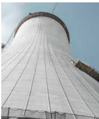
▲ Doka provided the formwork solution based on the Cooling-tower formwork SK175 for the construction of the 164 m high cooling tower of the coal power station Sostanj in Slovenia. The self-climbing system for pouring sections of 1.50 m high allow for precise forming with extremely short cycling times.
