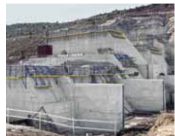
▲ The history of Doka is closely connected to the construction of power stations. Decades of experience in international power station projects, such as the Castrovido Dam in Spain, benefit Doka customers during implementation of their construction projects.
