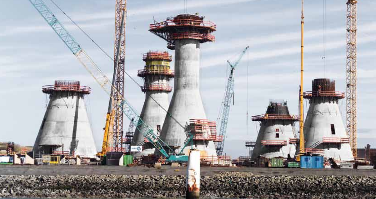
▲ Doka systems are used for foundations as well as towers during construction of wind mills, such as the offshore wind farm Thornton Bank in Belgium.
