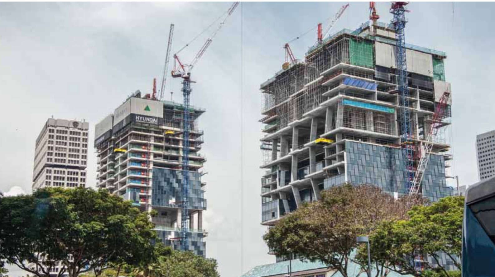
▲ Huge Mixed Development project in Singapore, The North and South Tower of South Beach Development
