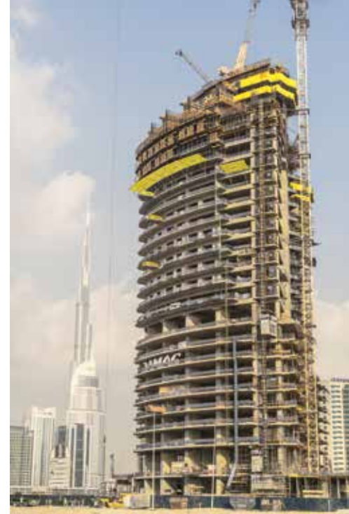
▲ Safety Nets are the ultimate fall arrest system for any highrise building.
