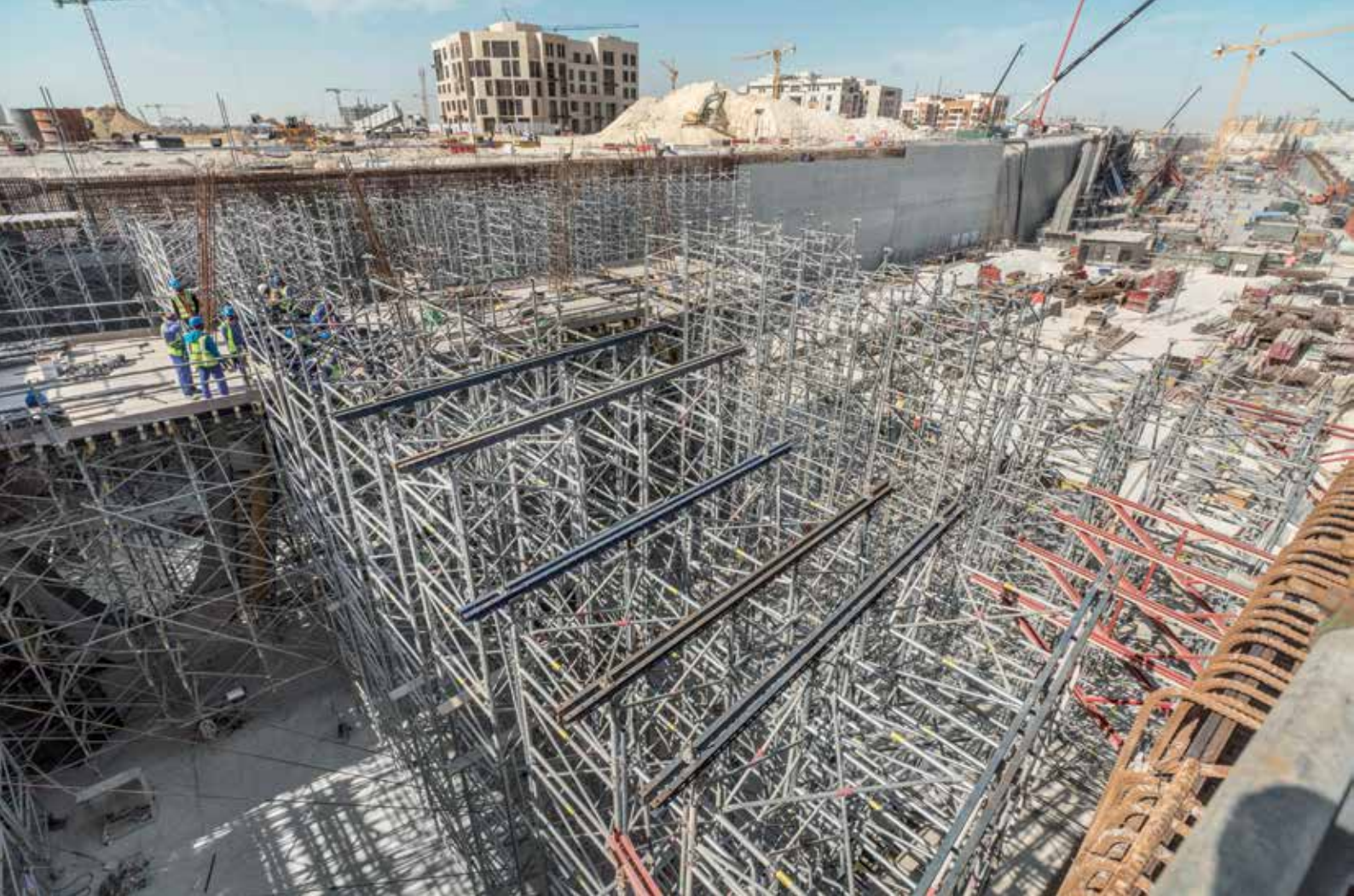
▲ Once complete, the pergola and bridge structure will become a central part of the Seef Lusail Waterfront.
