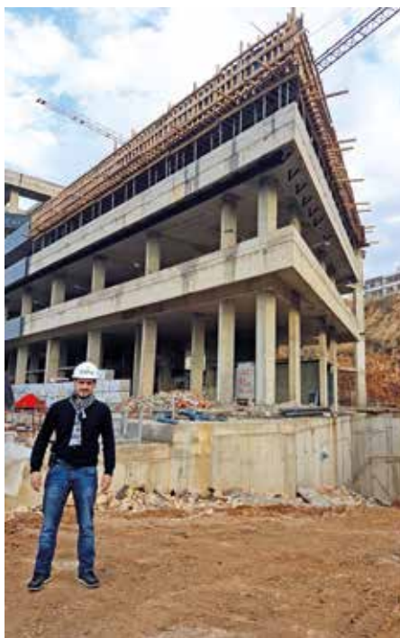
▲ The Danco Commercial Center (DCC) is being developed at a cost of $60 million.
