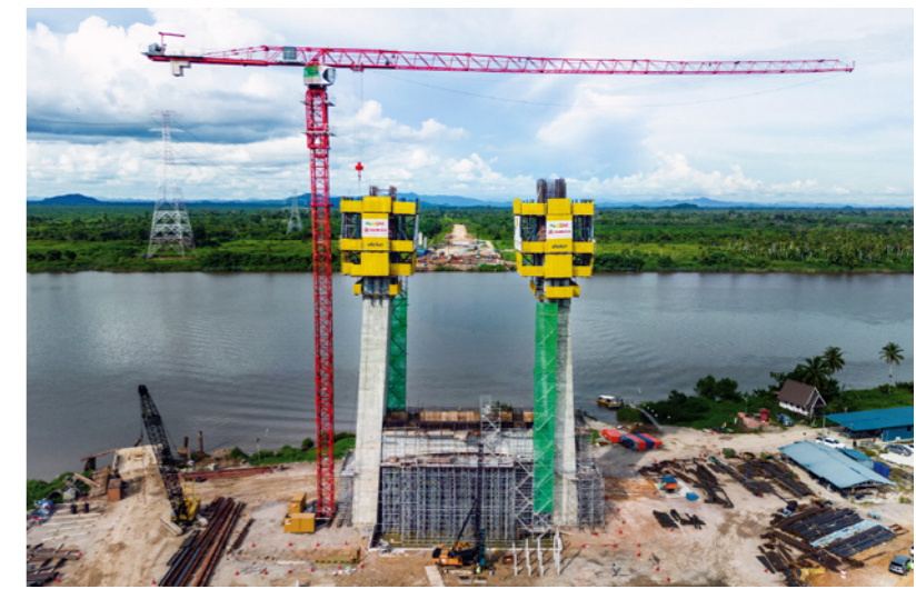
Pylons on the western banks of the Batang Lupar River to the southeast of Kuching.
