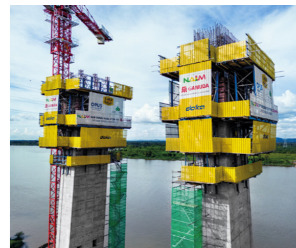
Doka's Automatic climbing formwork SKE100 plus have already saved months from the project schedule.
