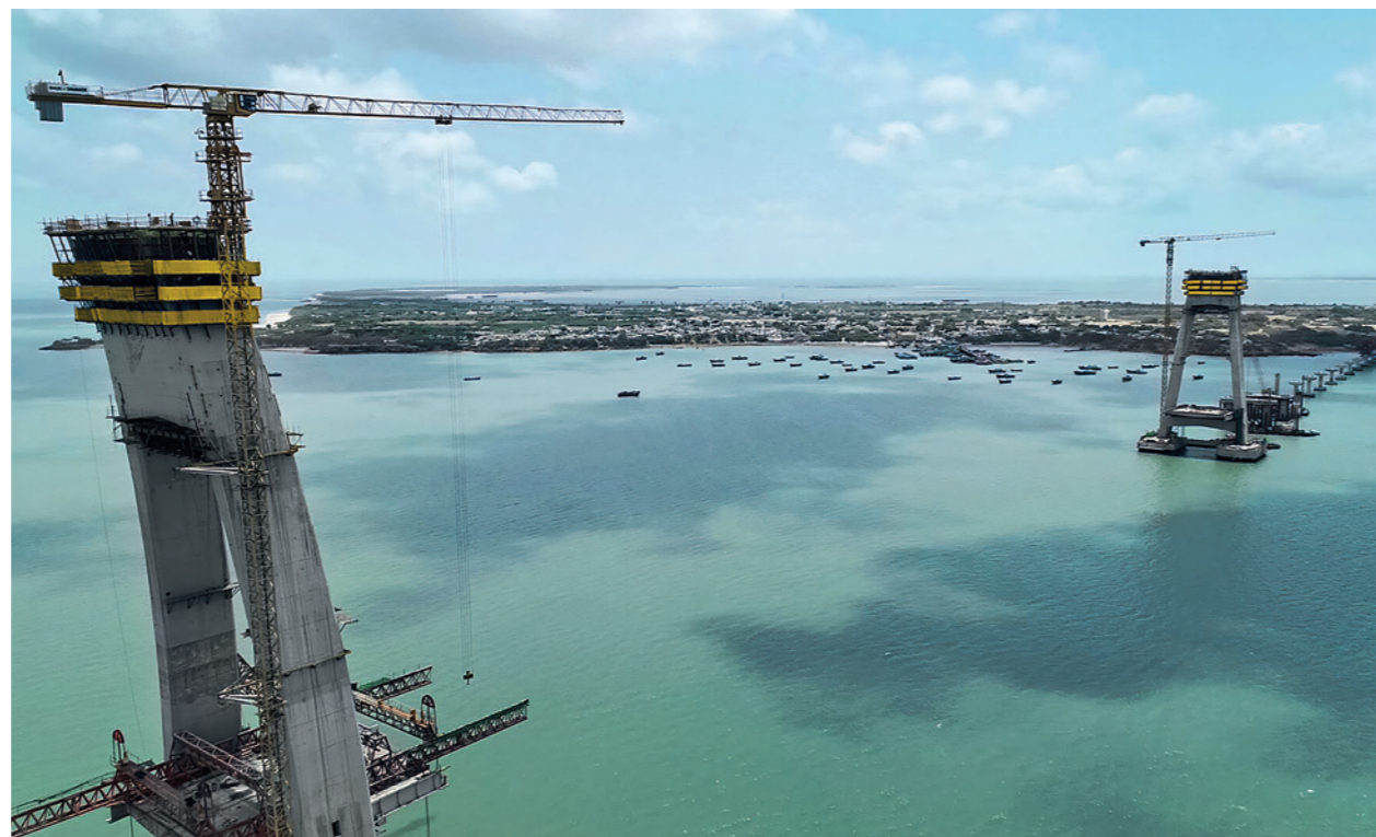
Pylon with self-climbing formwork at Dwarka Bridge Doka's crane-independent, self-climbing, structure-guided and all-hydraulic formwork solutions support the delivery of Asia's most challenging pylons and record-breaking bridges.
