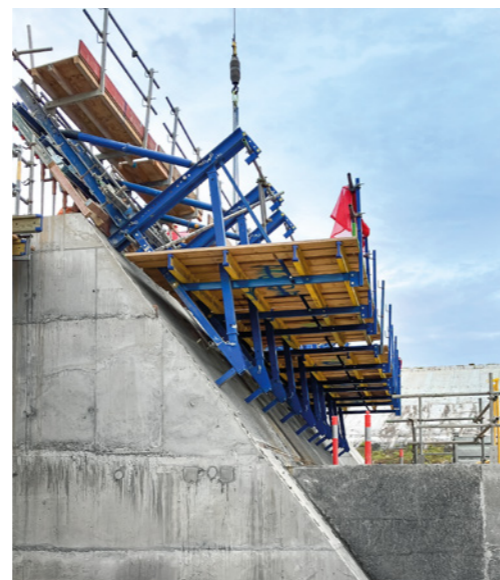
Taking place over 28 months, Doka's formwork solution for the 130,000 m 3 of mass and structural concrete.
