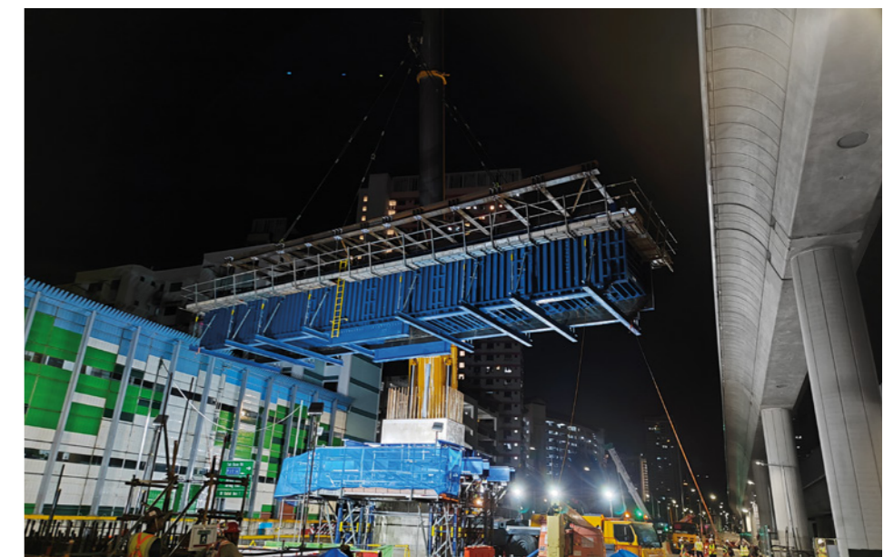
Doka's solution included crane-lifting its Steel Girder Formwork at night to avoid disruption to existing infrastructure.
